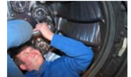
With Superbolt tensioners, joints in awkward positions in confined spaces can be tightened. This Francis wheel has regular maintenance requirements which became manageable with MJTs connecting the wheel to the shaft.
