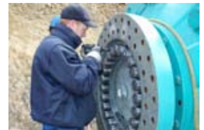
Flange coupling of the gear box on a wind turbine. An expansion bolt with integrated Superbolt technology is used to transmit the enormous torque. The solution is also compact and does not add a lot of weight, which was a requirement.
